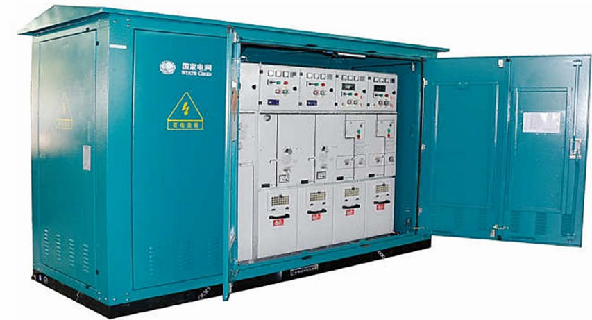
SF6 Insulated Ring Main Unit
